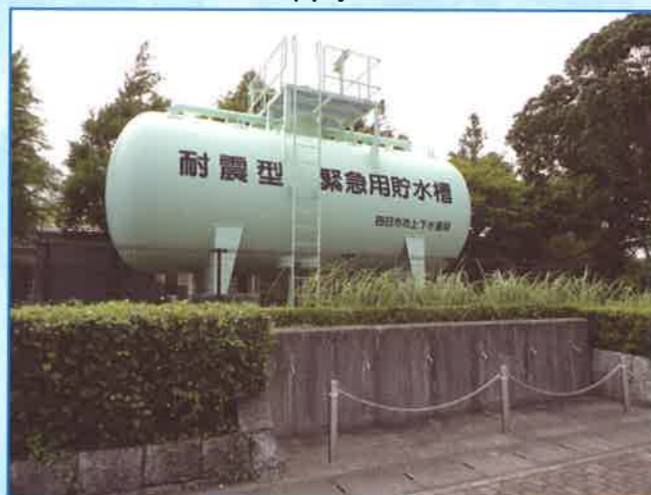
【Emergency water tank (above ground-type)】
