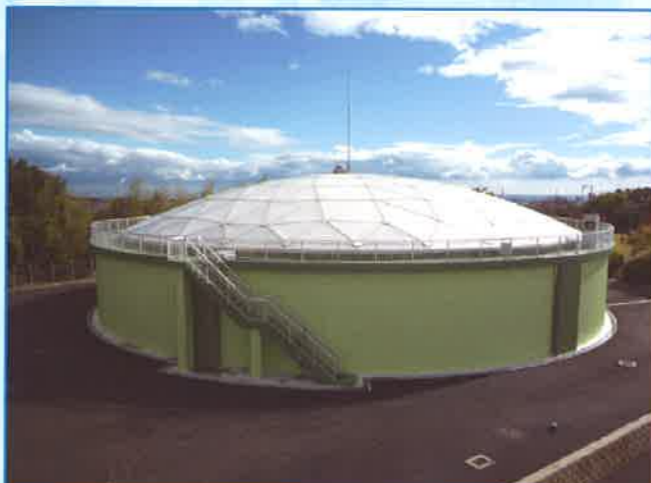
【Water storage tank (with emergency shut-off valve)】 In the event of a disaster, these installations supply drinking water.
